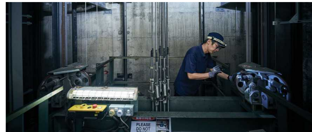
Lifts equipped with remote monitoring and diagnostics capabilities enabled predictive maintenance and improved lift performance.
